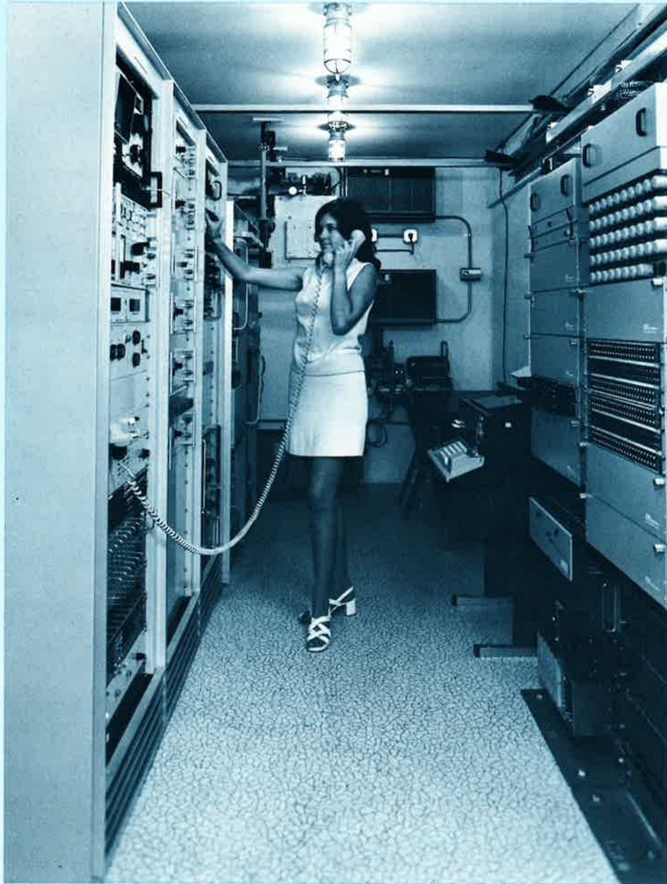
Interior view of Kwajalein earth terminal equipment shelter providing a complete redundant communication capability. This terminal was produced and installed by Comtech in 75 days in response to an urgent communication requirement.
